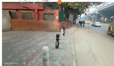
Inappropriate gap between bollards and absence of bollards at some places
