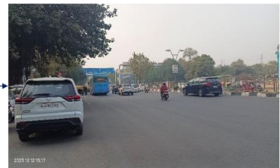
Absence of road markings, signages and speed control measures at the intersection.
