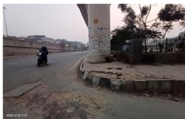
Obstructed pedestrian infrastructure
