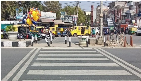
Inappropriate gap between bollards
