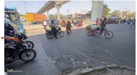
Damaged & uneven road surface and pedestrian infrastructure
