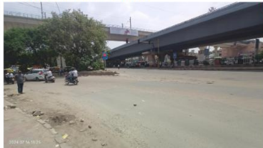
Absence of delineators, chevron and hazard markings
