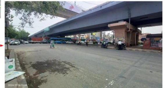
Absence of signages and speed control measures at the intersection.
