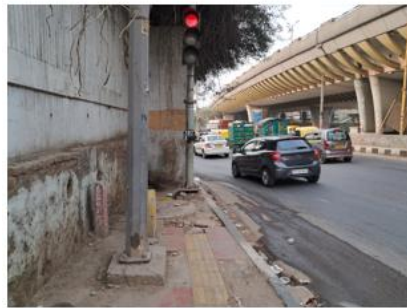
Damaged and obstructed pedestrian infrastructure on each arm
