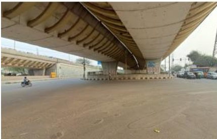
Absence of delineators and reflectors on the median and carriageway edges.
