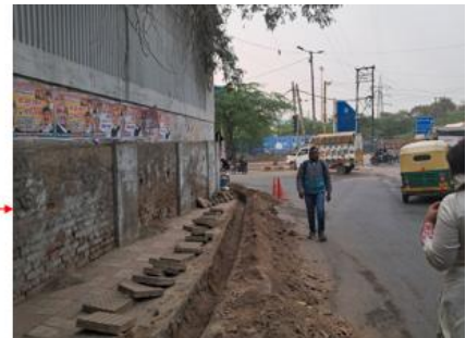
Lack of pedestrian path at the construction site.
