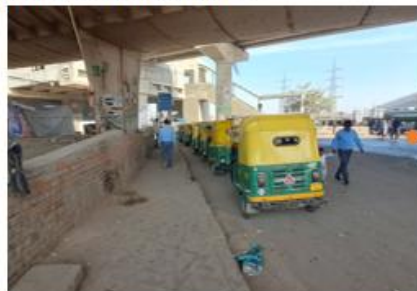
Damaged & uneven road surface and pedestrian infrastructure.
