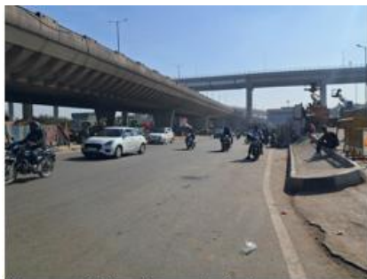
Absence of delineators and reflectors on median and carriageway edges.
